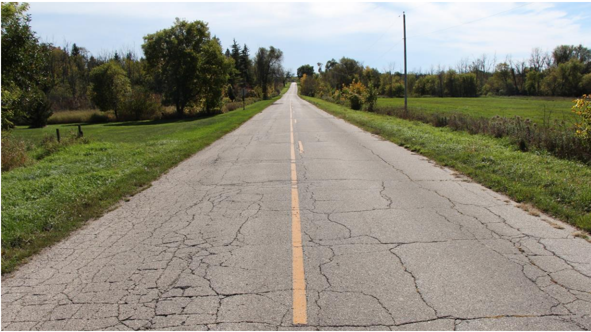
The segment of demonstrates a PASER rating of “2-3” (2021) due to the failed asphalt surface. insufficient drainage.
