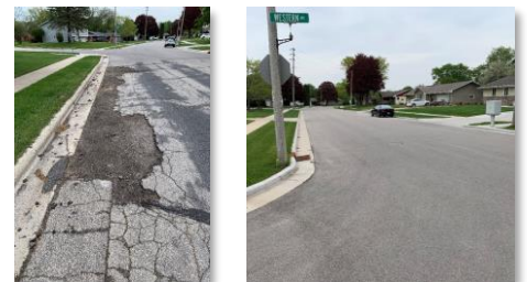
Existing pavement condition is one key factor that was considered during the planning process.
